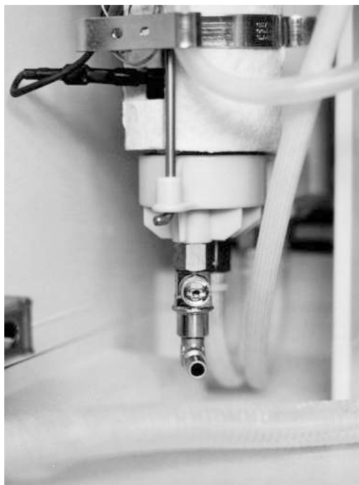
Figure13: Steam generator emptying
